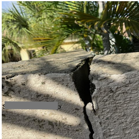
Level 2 - Significant Concern
