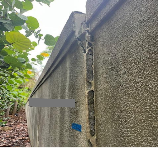
Level 1 - High - Structural Concern.
