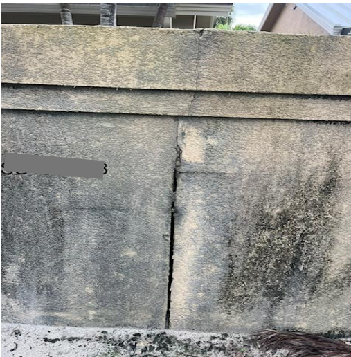
Level 3 - Medium Concern. Repair asap
