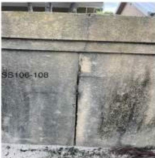
Level 3 - Medium Concern. Repair asap
