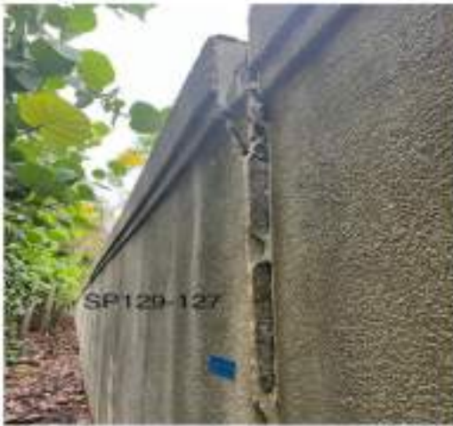
Level 1 - High - Structural Concern.
