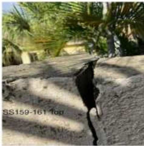
Level 2 - Significant Concern
